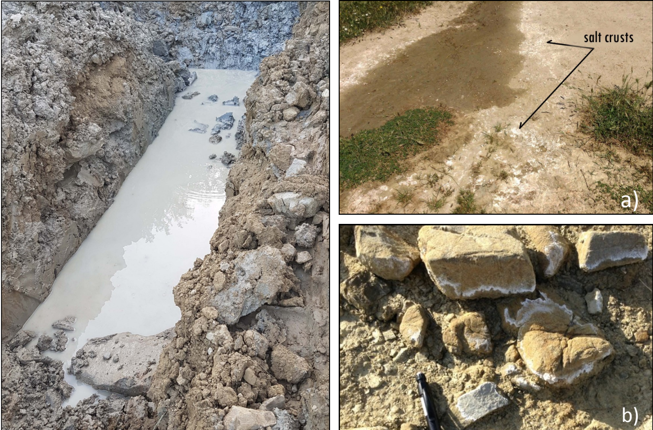
Fig. 8, left -The large flow of La Rossa turbid groundwater after a trench excavation.
